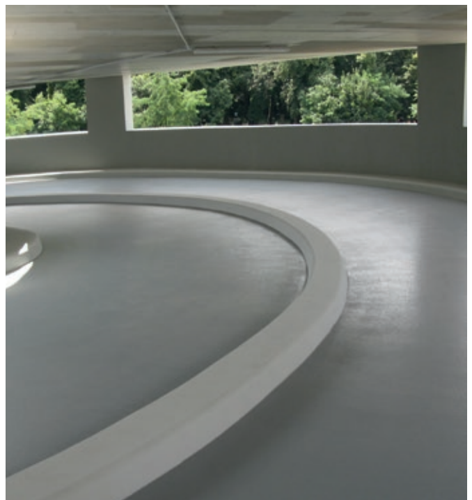
Areas exposed to heavy use of any de-icing agents (salts), e.g. parking decks
